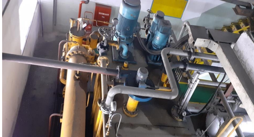
Gambar 2.9 Auxiliary Oil Pump
