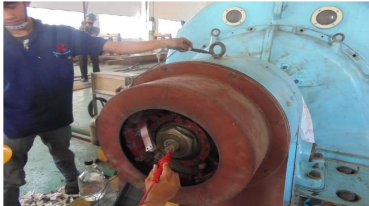
Gambar 2.18 Megger Rotor Generator STG PT. Soci Mas
