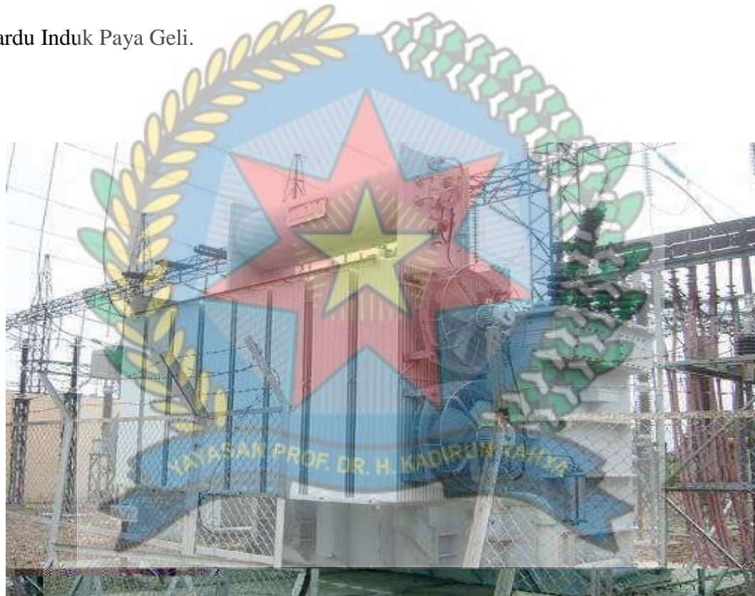
Gambar 3.2 Transformator Daya 1 (TD 1)
