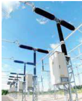
Gambar 2.10. SF6 Gas Circuit Breaker
