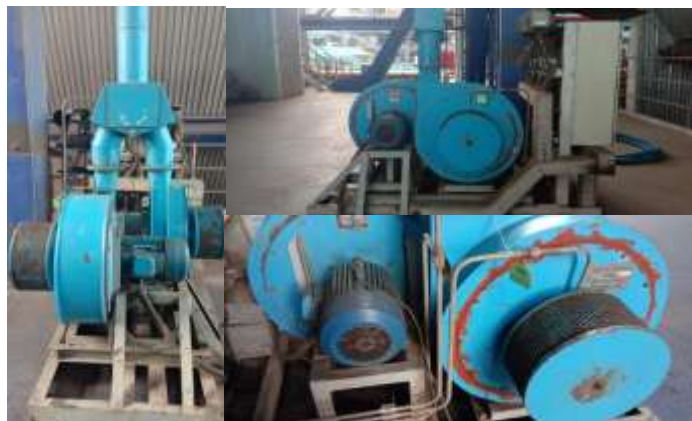
Gambar 2.20 Scanner Cooling Air Fan Sumber: Penulis, 2020
