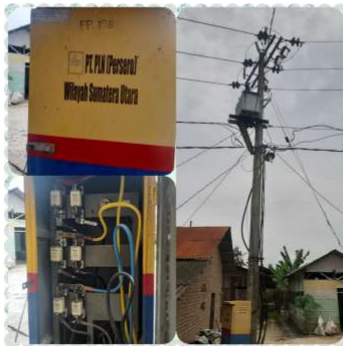
Gambar 4.2 Gambar Trafo PR198
